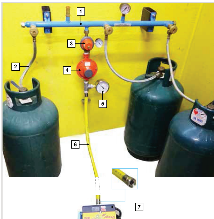
Rampa gás - GPL/LPG
